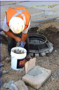
Darrin Sharp of Mark One Restoration Services of Detroit replaces some of the brick pavers in front of the depot.
