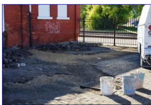
Installation of storm drains at the depot (top) and the express building (bottom)
