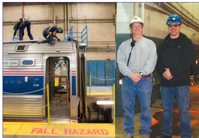
Crew at the Ivy City Maintenance Facility mounted the roof antennas. Foreman Ron Wallace & Electrician Scott Sebby were part of the crew at the 14 th Street Facility that did the installation.
