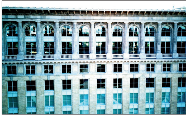
The upper floors at Michigan Central Station where the new NoMad Hotel will be located. (Gary Melford photo)
